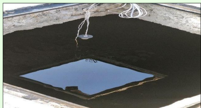
Sensor tank overflow
